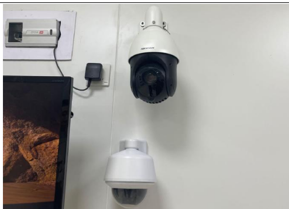
(机房内摄像头 3)
