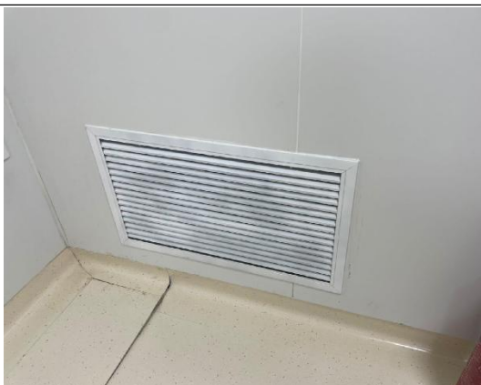
(机房内排风口)
