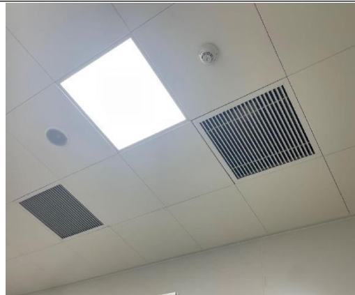
(机房顶部新风口)
